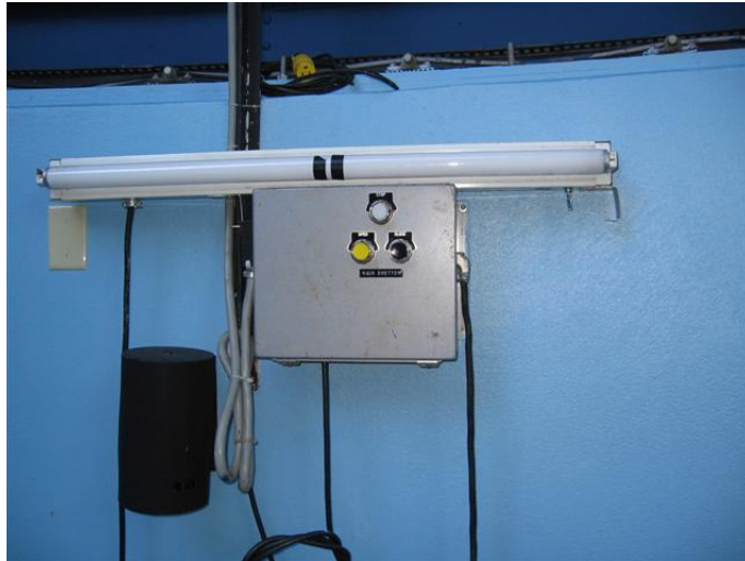
Figure 1: Dome shutter control panel with pushbutton switches to open and close the shutter.
