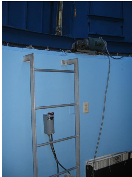
Figure 2: Dome motor control switch and ladder. Note the west dome motor in upper right of photo.
